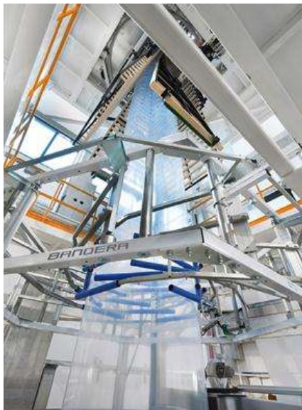
Figure 7: Five layers Coextrusion line TechnoFlex Plus of Bandera [taken from "Film, Sheet and Extrusion" magazine, November 2016].
